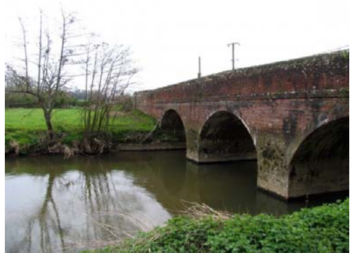
Shopham bridge viewed from the south bank on the 'Shopham Up' side.
